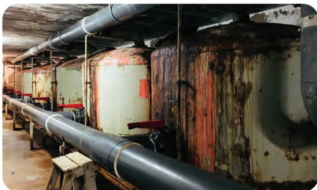
Corroded metal fabricated filters
