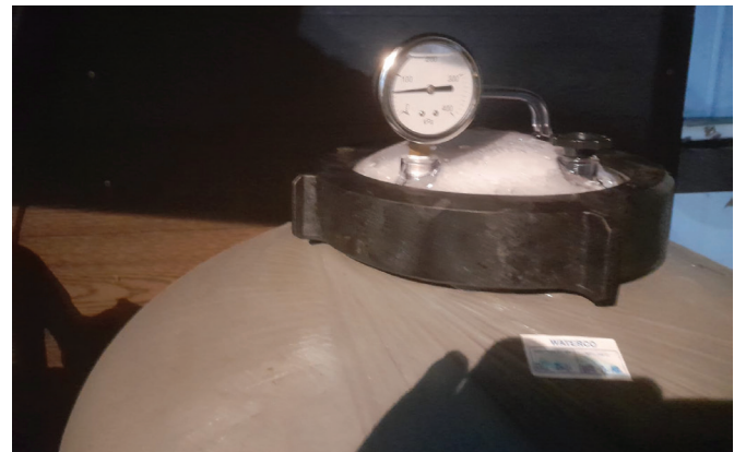
Pressure gauge at the top of ASM600 for monitoring
