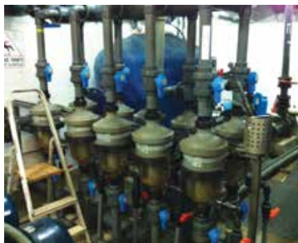
60 of Waterco's MC16 MultiCyclones that were used to effectively and efficiently remove the sand from the water before it was pumped into the pools.
