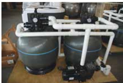
Hydroxypure sanitisation system, two Micron S702 fibreglass filters, a Supatuf 250 pump and an Electroheat heat pump is installed on every pool.
