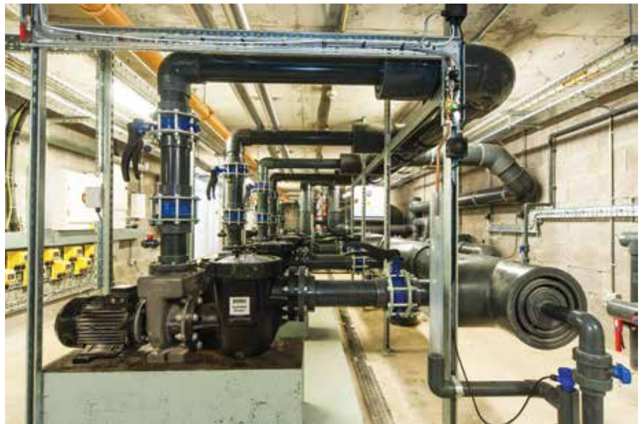
▲ Four 7Hp BH5000 Cast Iron Pumps were installed for the main pool and two Hydrostar 6HP pumps for the children’s splash pool.
