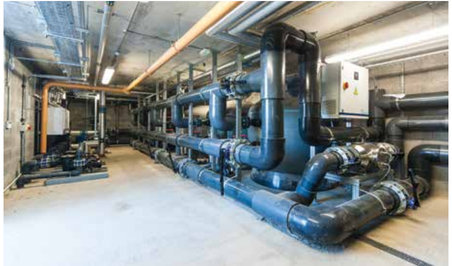
▲ Five SMD1800 Micron commercial sand filters were installed for the main pool and one SMD1800 Micron commercial sand filter was installed for the children’s splash pool.
